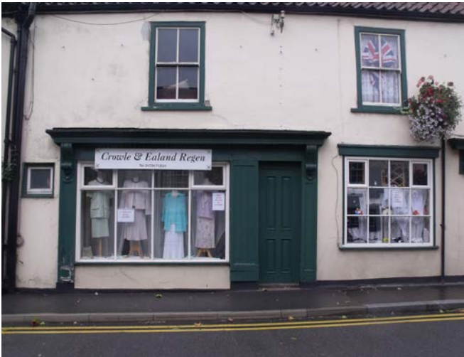
Figure 5 This shopfront has been built in timber and is in character with the traditional building and the conservation area.
